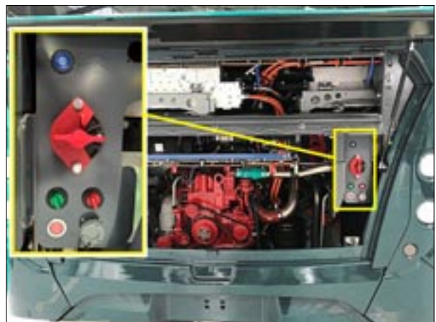
Engine Bay Switches
