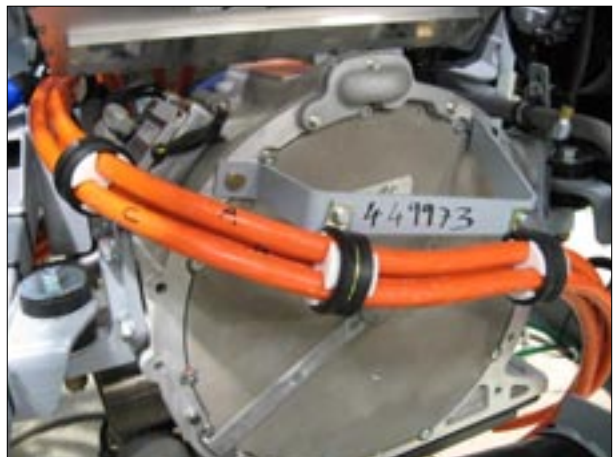
High voltage cables in orange coloured loom
