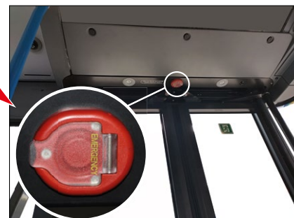
Internal Emergency Exit Button
